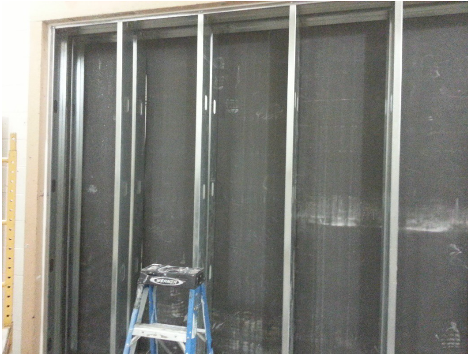
Figure 3 – Detail of studs and Wall Blokker installed on studs on one side.
